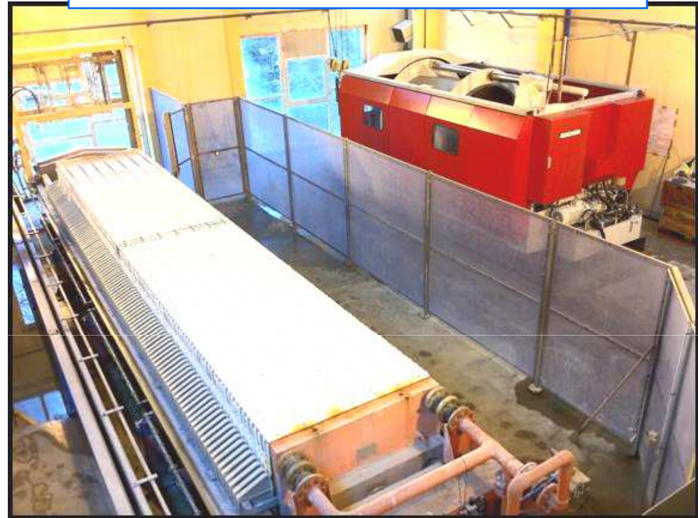
5,000 L chamber filter press and HPS 3007
